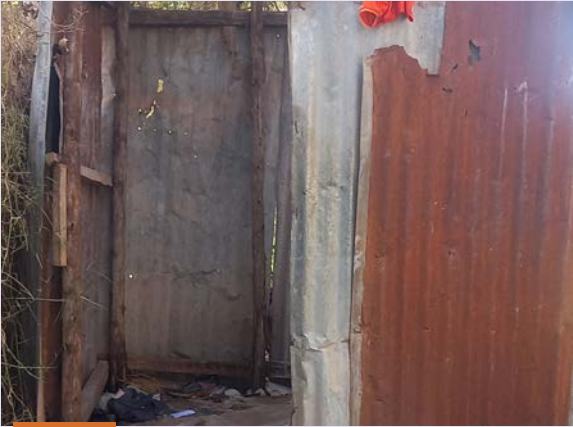
State of the old bathroom used by the boys.
