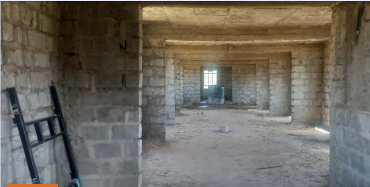
state of the old incomplete upper dormitory.
